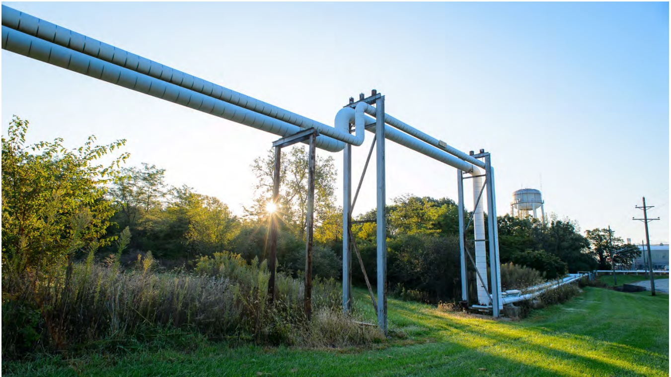
Figure 23: Maintenance of Steam Distribution Piping Improves Resilience of Campus Heating System
